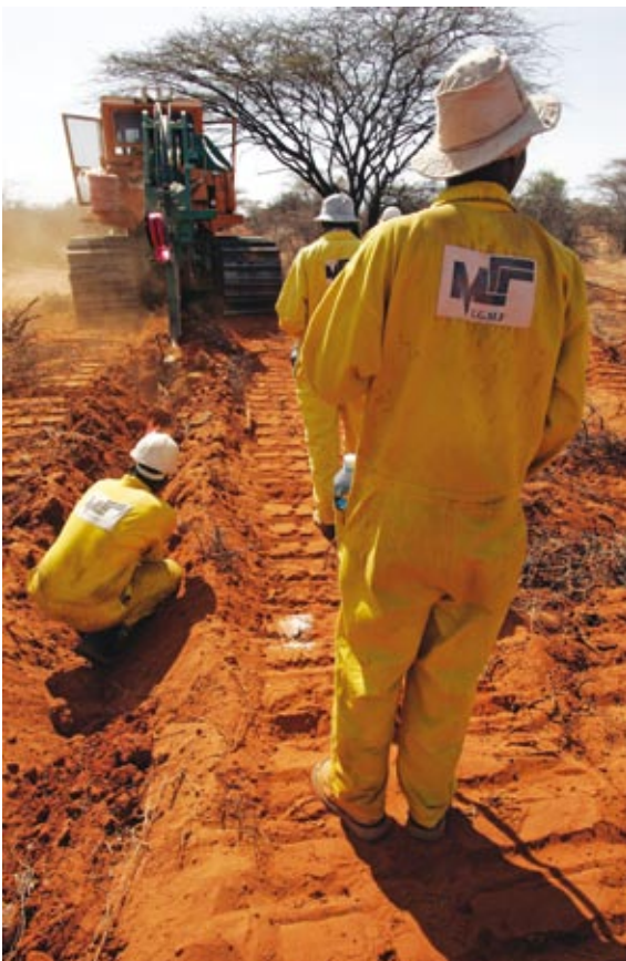
A team of engineers lay fibre optic cables, as part of a government project to provide internet and telephone services, at Seredupi, 450 kilometres north of the capital city, Nairobi, in Kenya.
